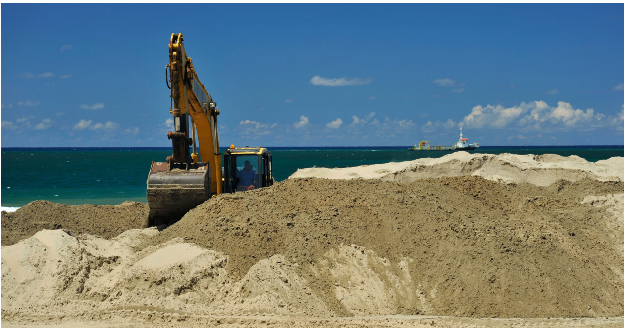
Mechanical excavation of sand to manage beach erosion and sea level rise, Golden Mile waterfront, Durban, KwaZulu-Natal, South Africa. Frank Kahts Durban
